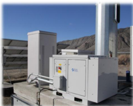
Hybrid DC Generator Extreme weather Remote monitored
